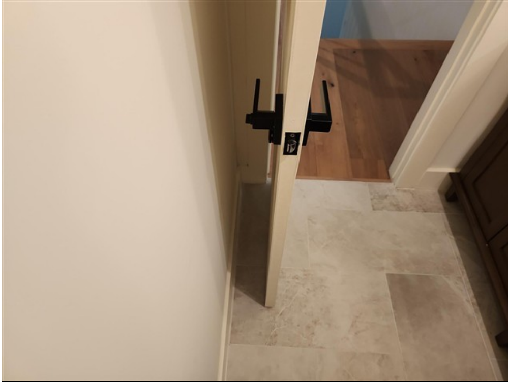
G. Example of missing doorstops
