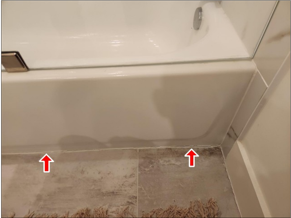
A. Caulking improvements needed at the tub to floor transitions
