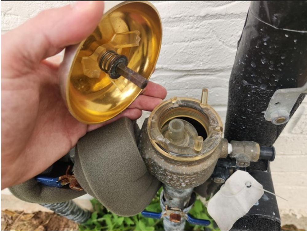
A. Vacuum breaker broken
