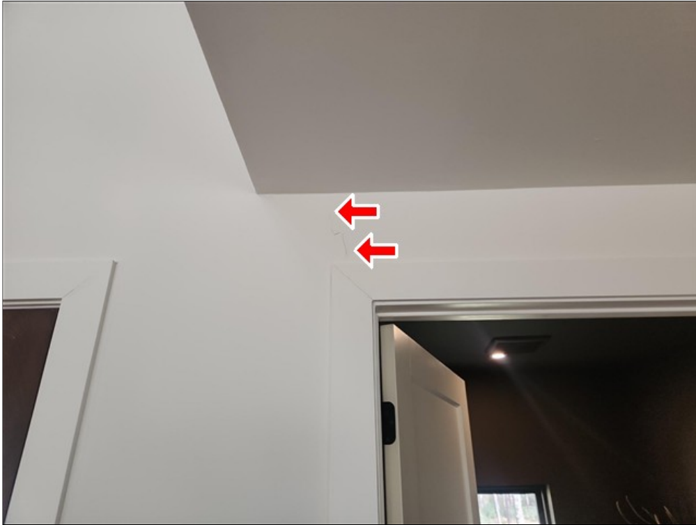
E. Drywall crack in wall above powder room door
