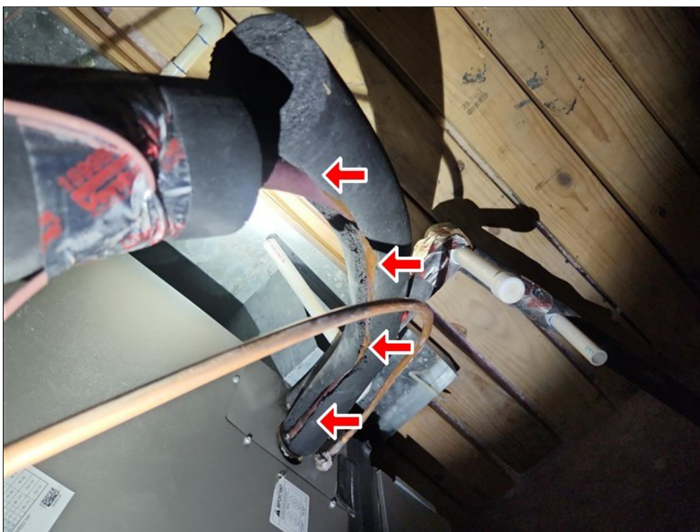
B. Insulation improvements needed at refrigerant line in attic
