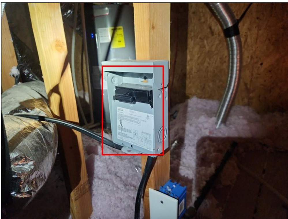
B. Cover plate missing for disconnect
