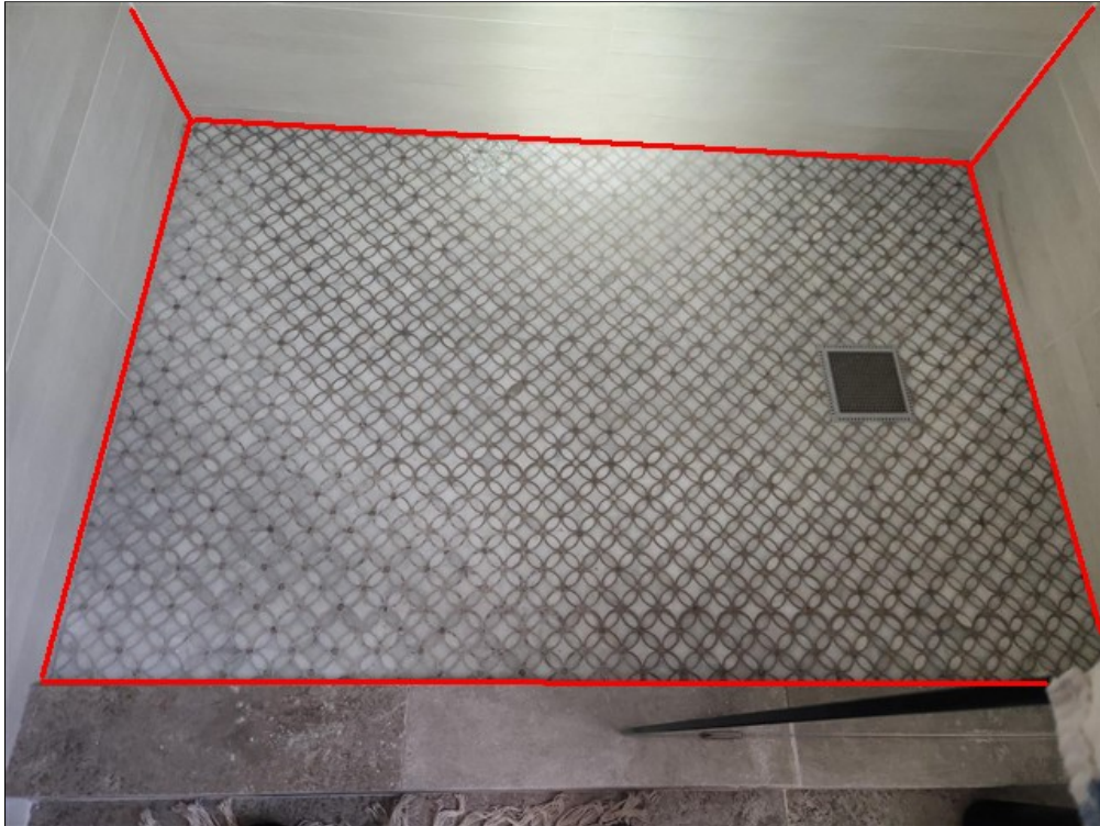
A. Caulking improvements needed in shower enclosure
