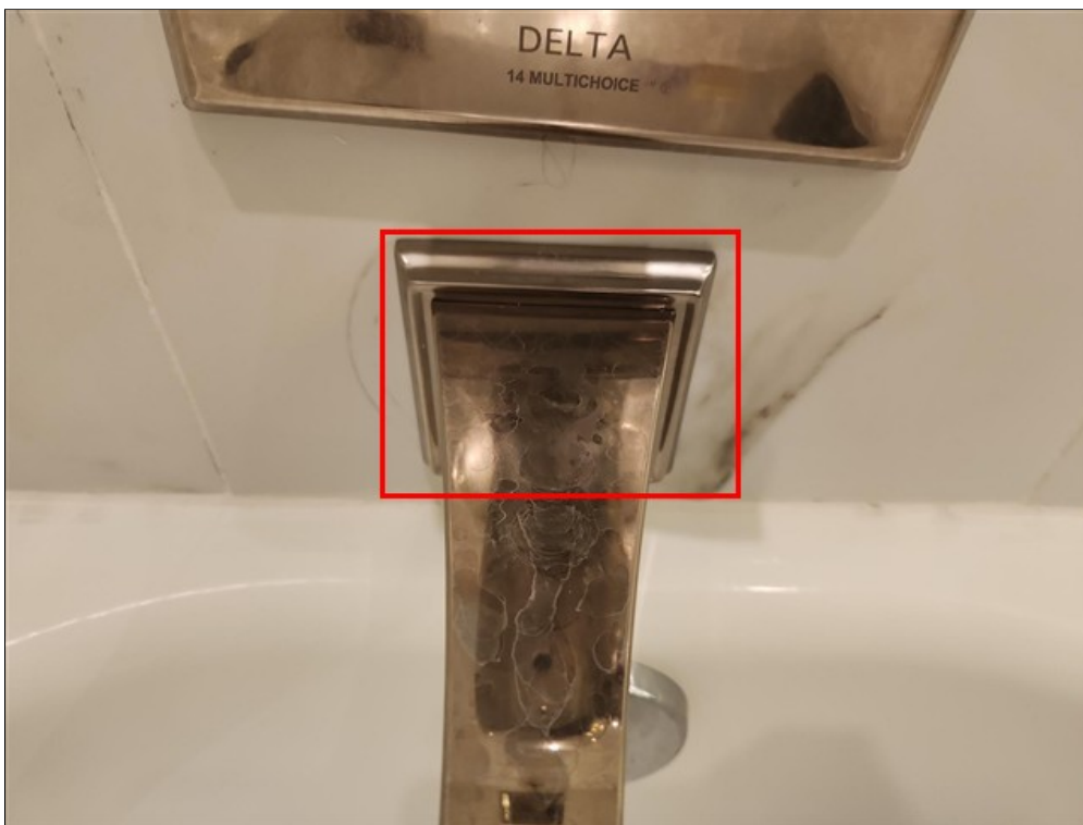
A. Caulking improvements needed around base of bathtub spigot
