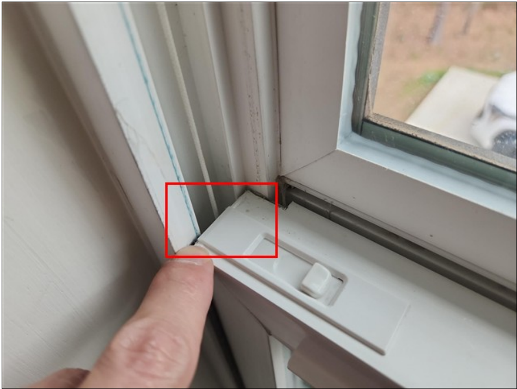
H. Far left window in second level right guest bedroom does not latch on left side
