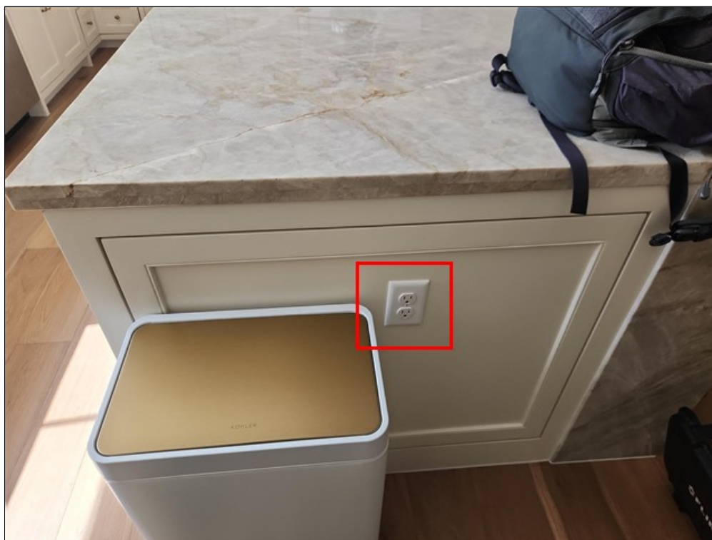
B. Receptacles installed in ends of kitchen island - also not GFCI protected
