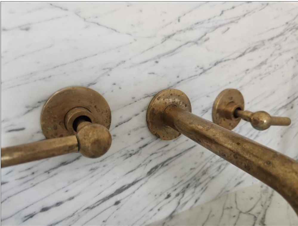
A. Corrosion observed at sink faucet and water valve handles
