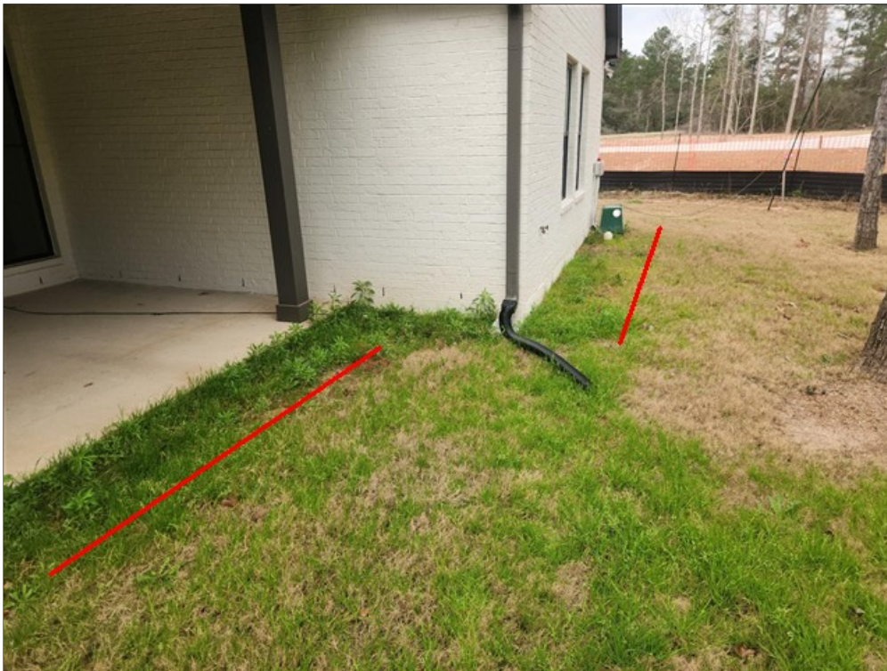
B. Photo showing area in need of grading improvements
