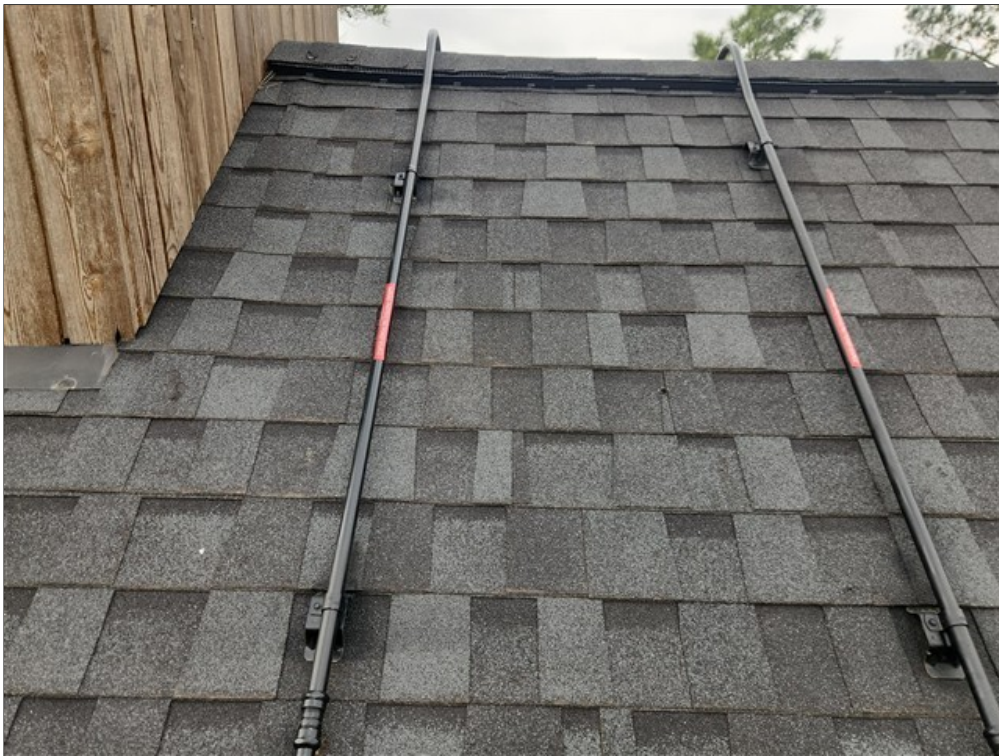
C. Areas where shingles are missing notable amount of their granules
