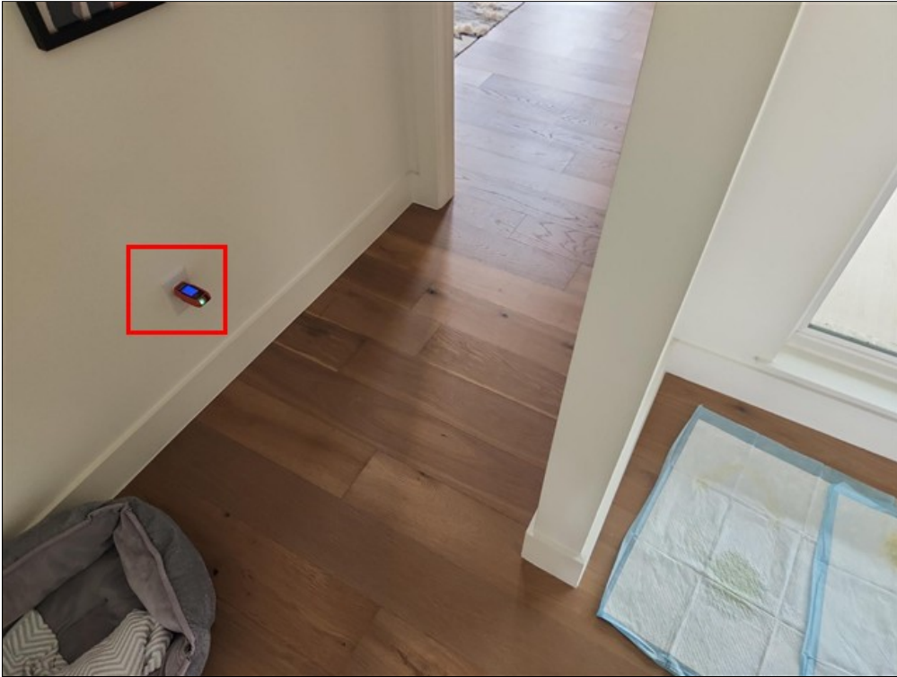
B. Some receptacles inside and outside of master bedroom have varying voltages
