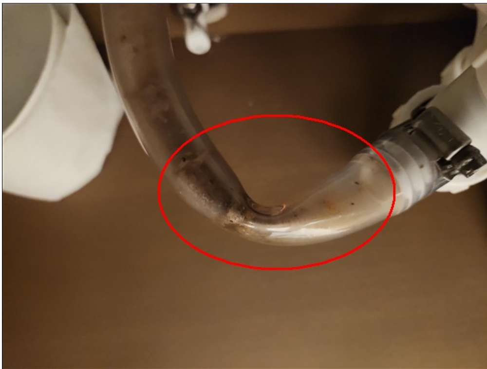
A. The primary condensate drain line pinched and clogged
