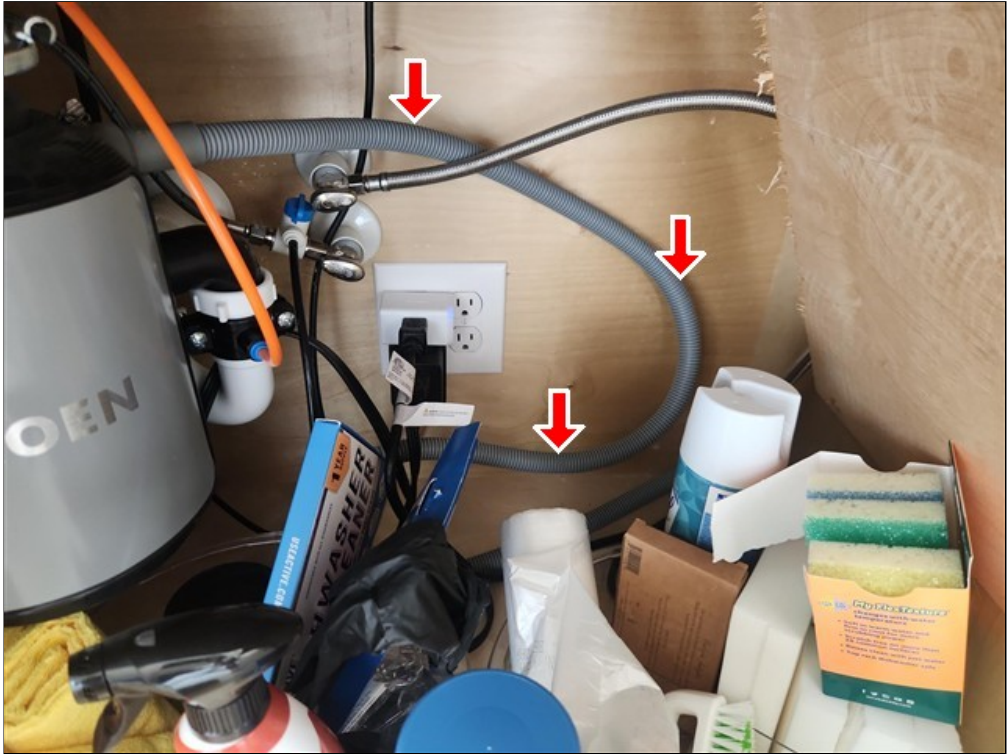
A. Dishwasher missing high loop
