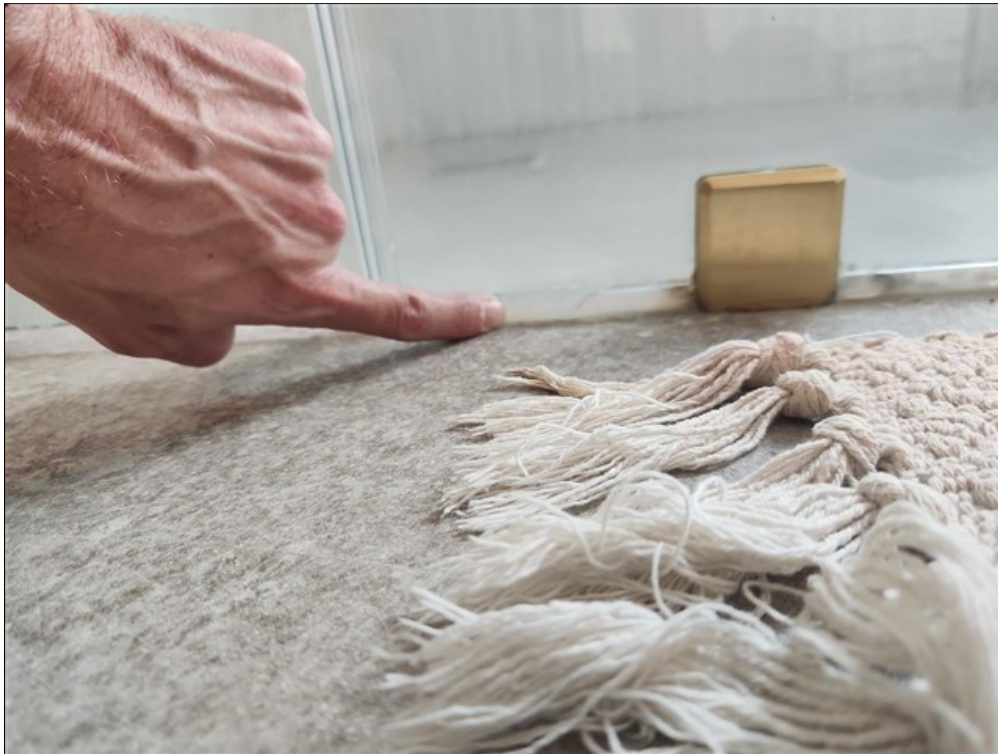
A. Gap between shower enclosure glass and floor approximately 1 inch - too large to be filled with caulking
