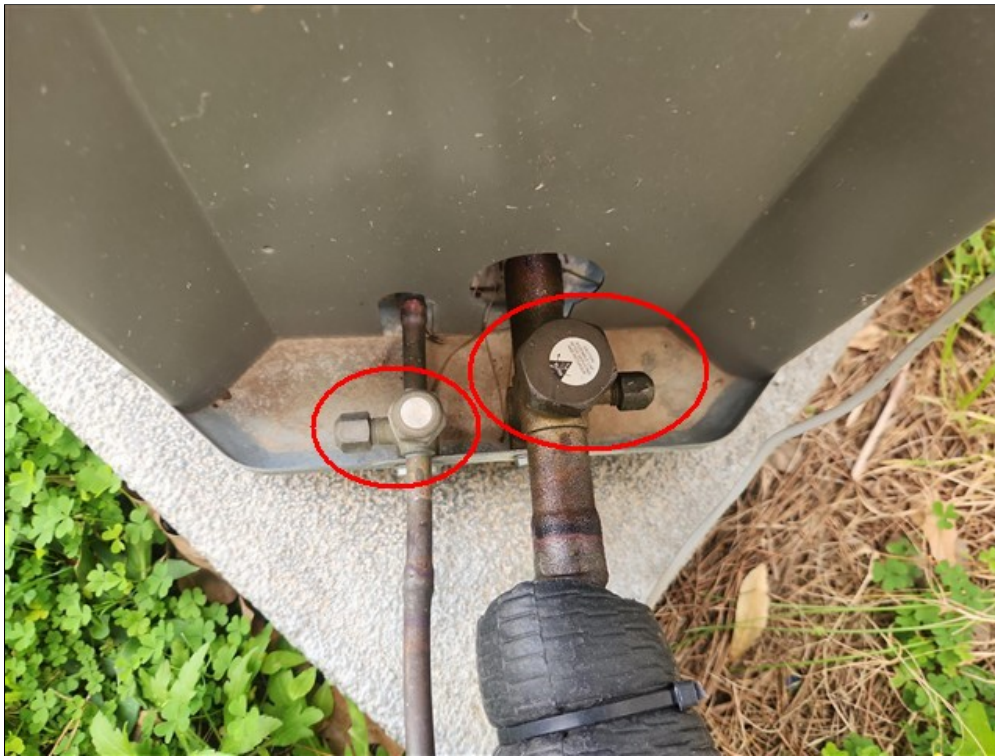
B. Locking caps missing at refrigerant ports
