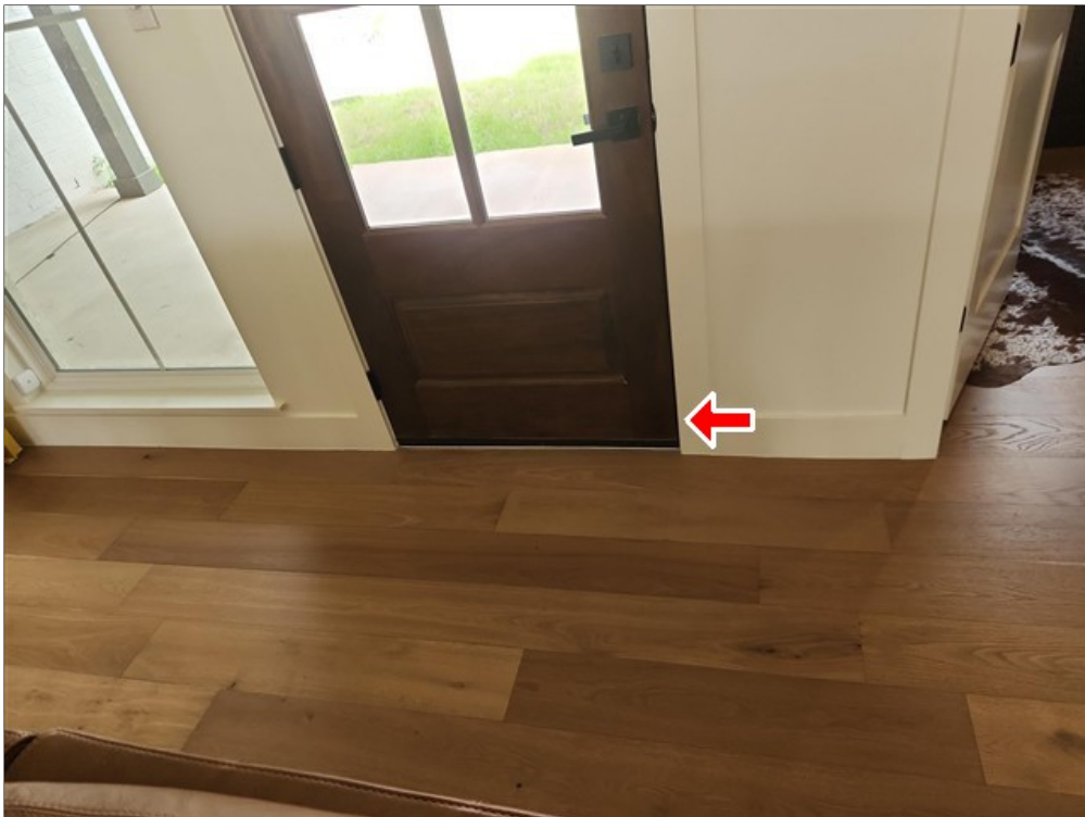
G. Rear exterior door rubs at jamb/bottom when operated
