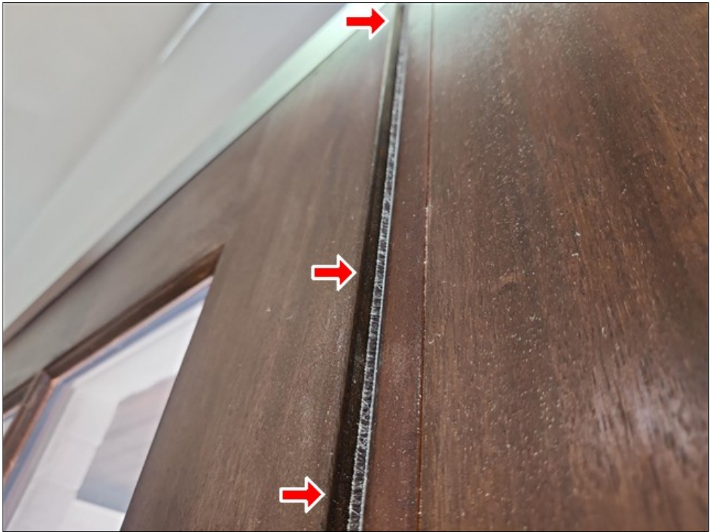
G. Exterior door at front of home appears to not be square with frame
