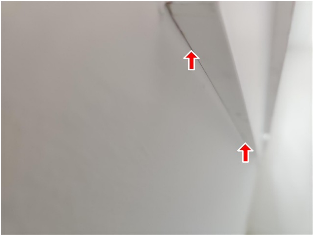
E. Example of caulking improvements needed at underside of window stool trim throughout the home
