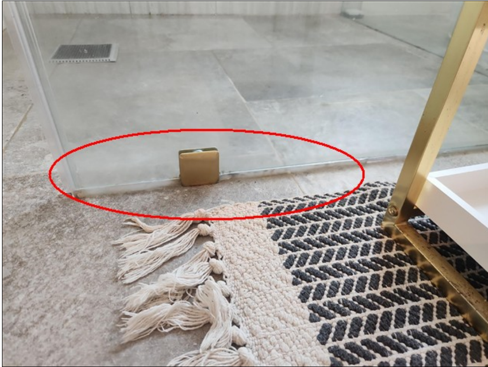
A. Leak at bottom of shower glass where caulking is filling 1 inch gap
