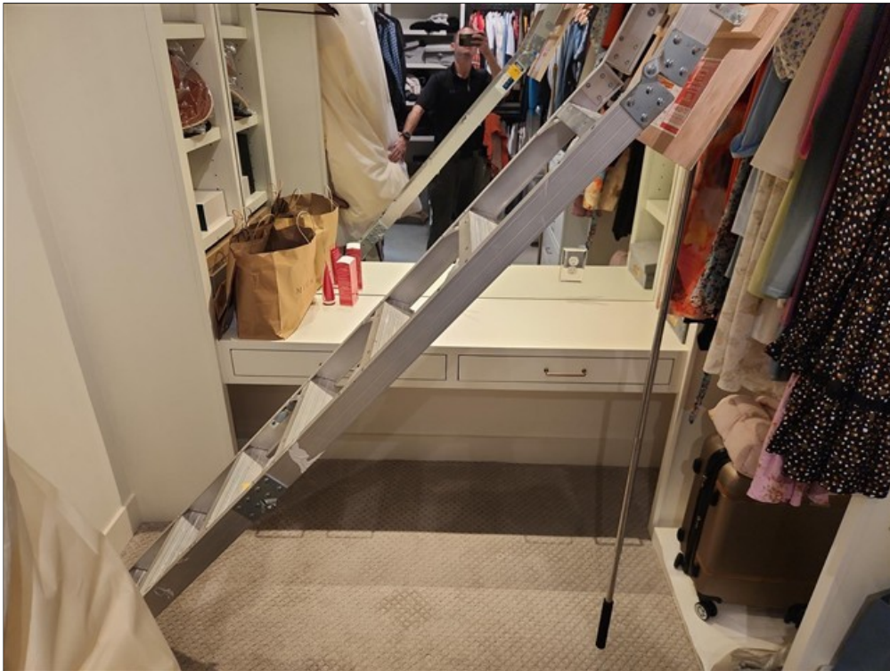
D. Attic pull down ladder in master closet is improperly installed/improper length
