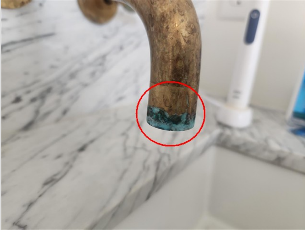
A. Corrosion observed at sink faucet
