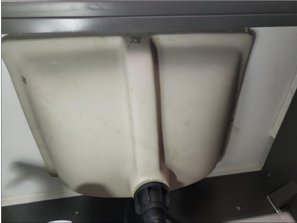
A. No clips/braces installed to secure undermount style sink to underside of countertop
