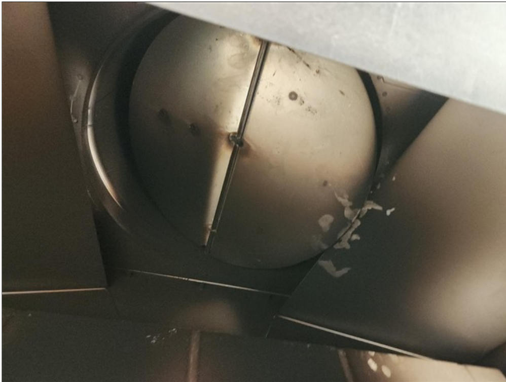
J. Fireplace missing damper stop
