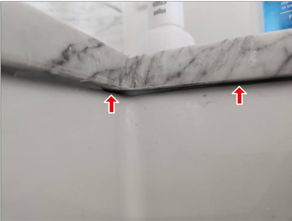
A. Caulking improvements needed at undermount sink to countertop transitions
