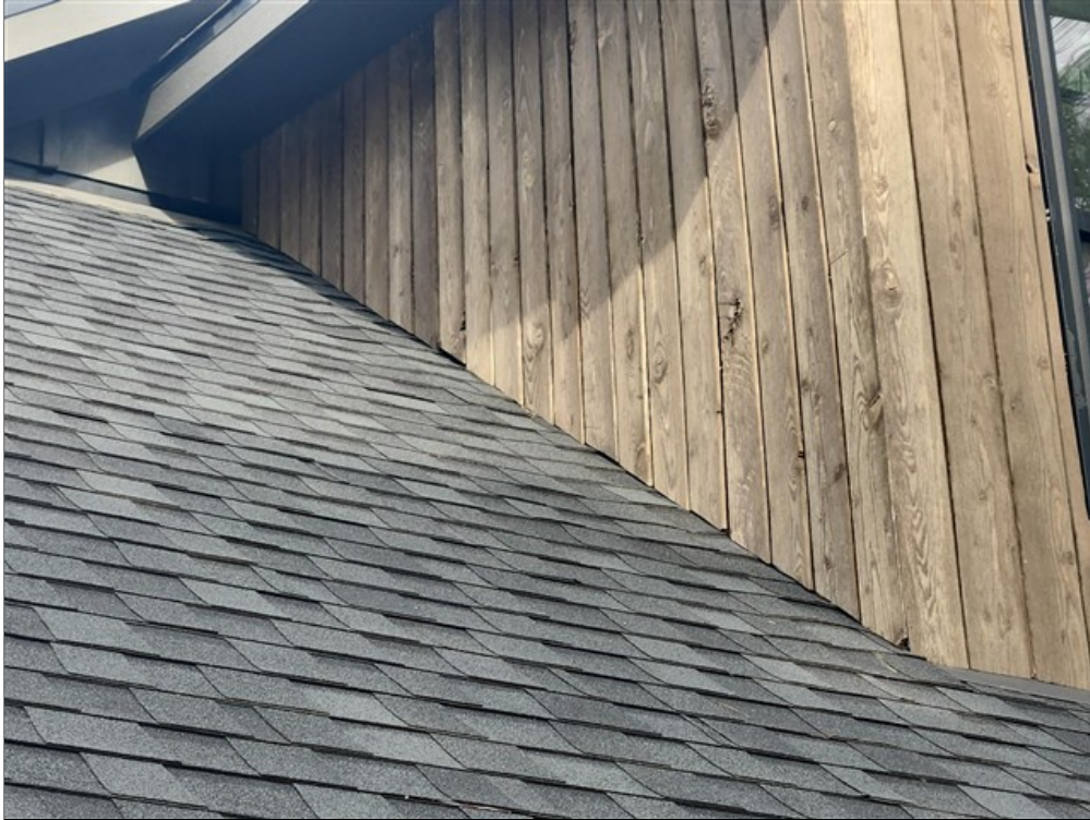
C. Photos showing wood siding has inadequate clearance from shingles in several locations
