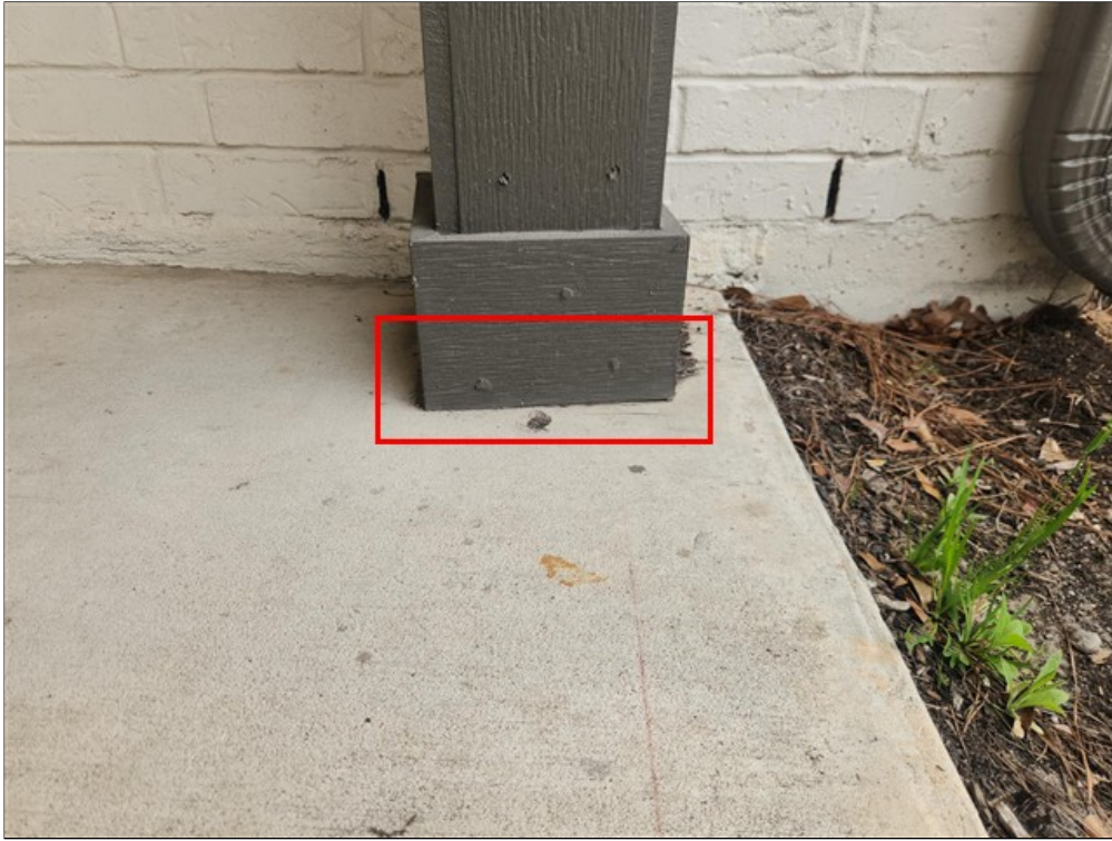
L. Trim at front porch columns in direct contact with concrete flatwork
