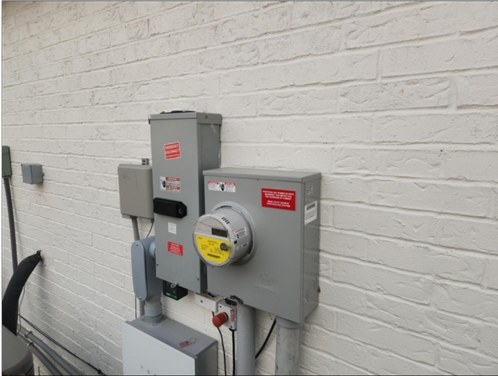
E. Caulking needed at top and sides of meter enclosure and main breaker
