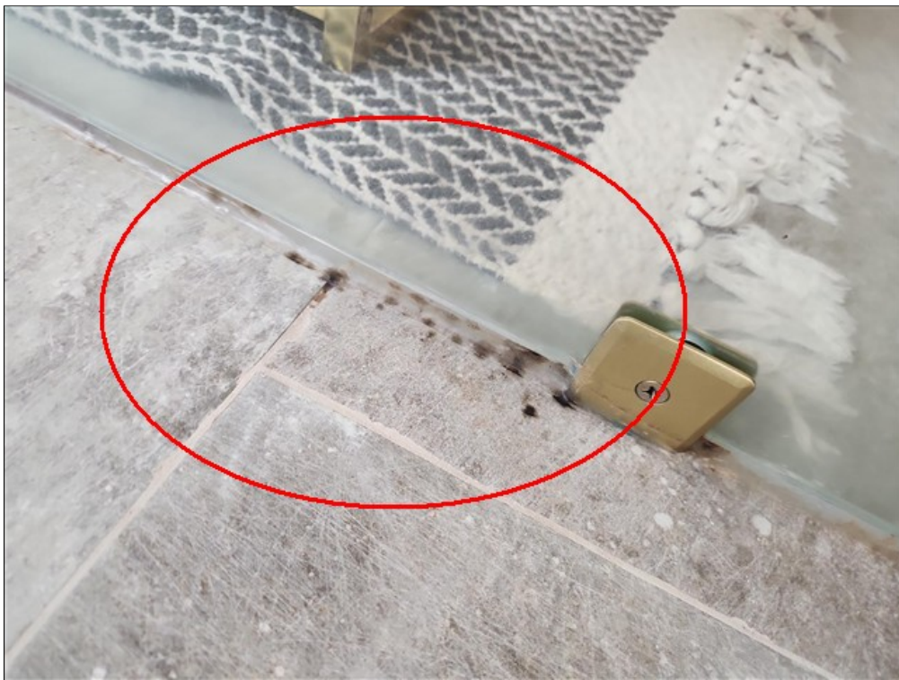
A. Mildewed caulking at shower glass to floor transition
