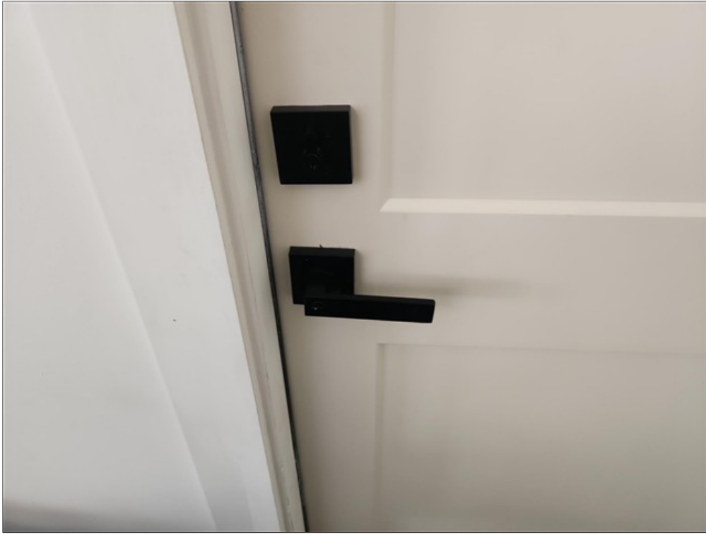
G. Door handle at occupant garage door loose
