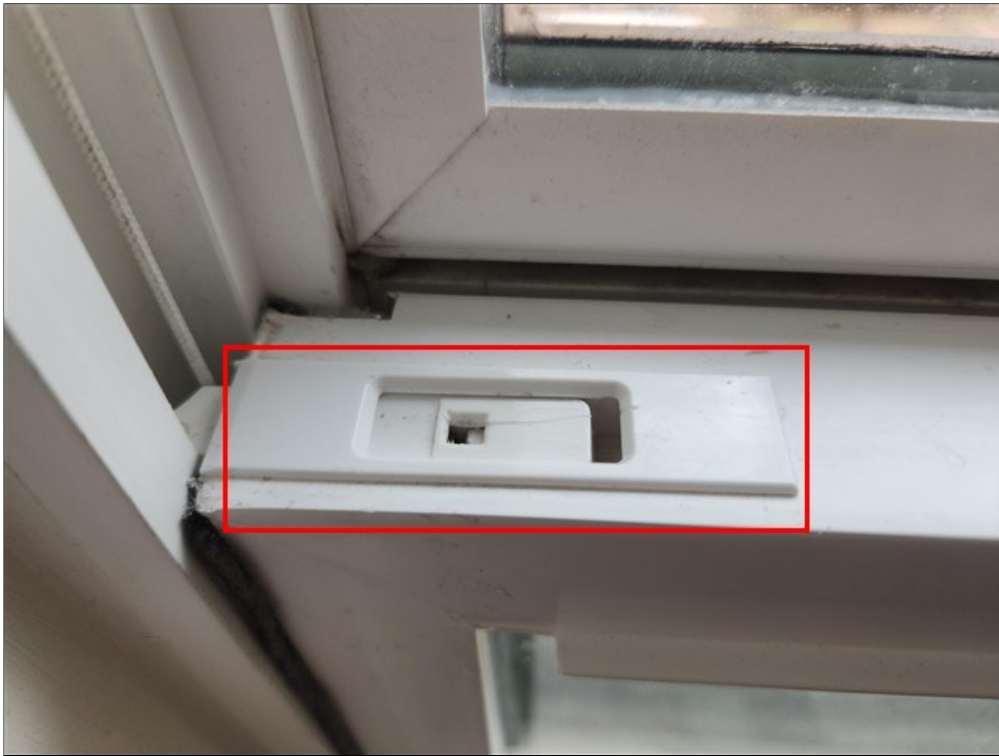
H. One latch missing at second level right guest bedroom right window
