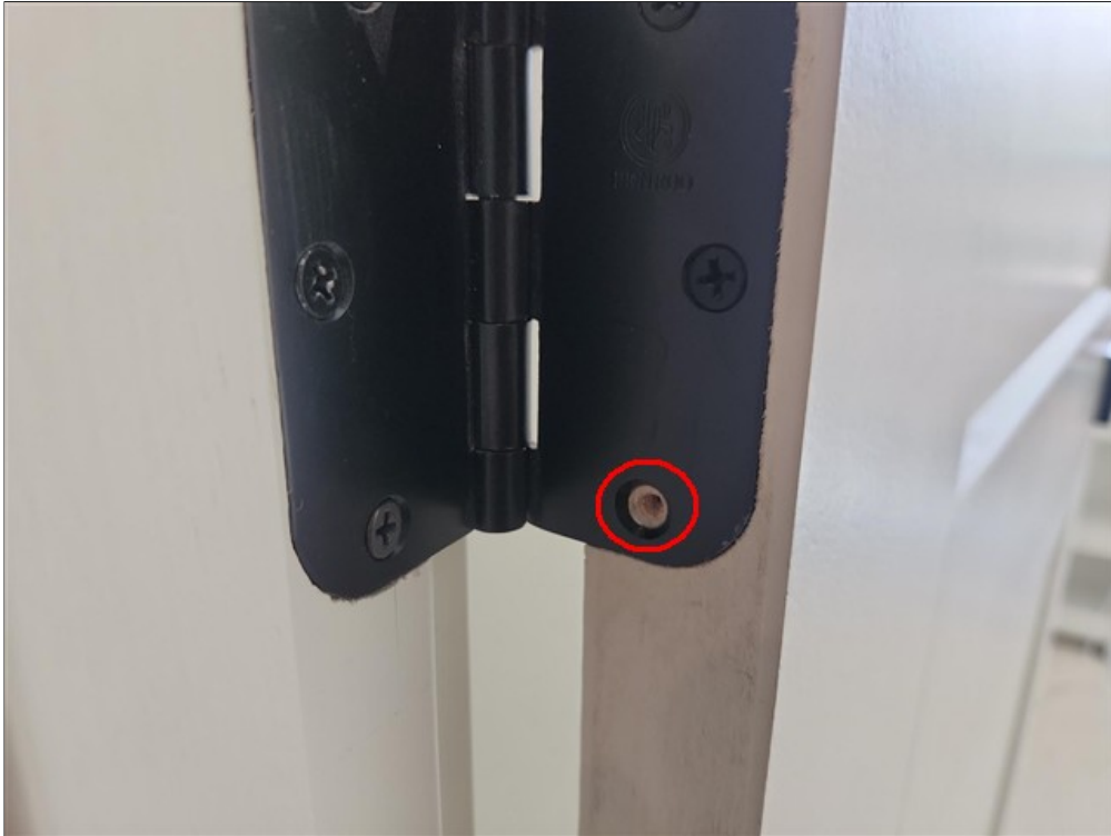
G. Second level front guest bedroom door missing hinge screw
