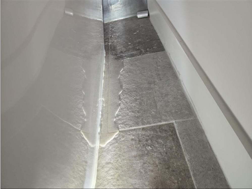
A. Water leak at glass panel of shower enclosure
