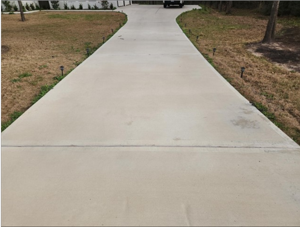
L. Photos showing two concrete driveway pads cracked across entire pad
