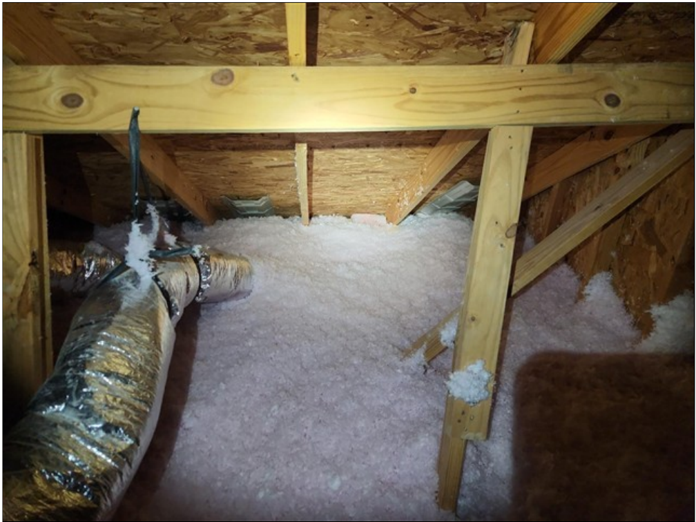
D. Baffles missing in attic
