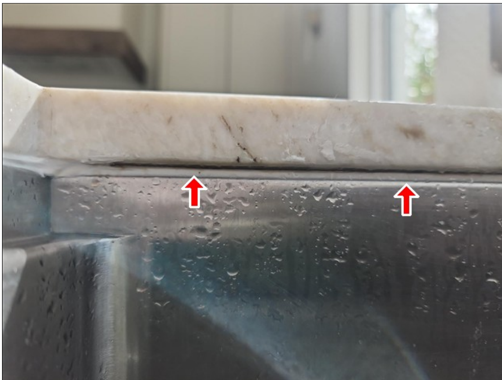
A. Caulking improvements needed at undermount sink to countertop transition
