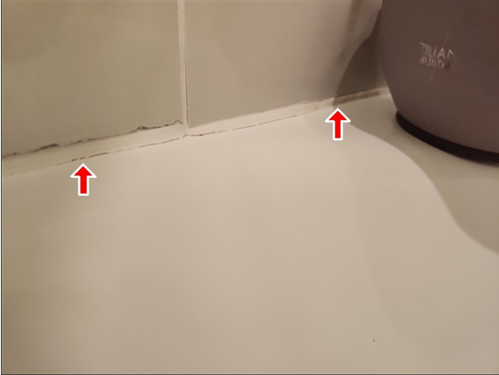
A. Caulking improvements needed at the shower wall to tub transitions
