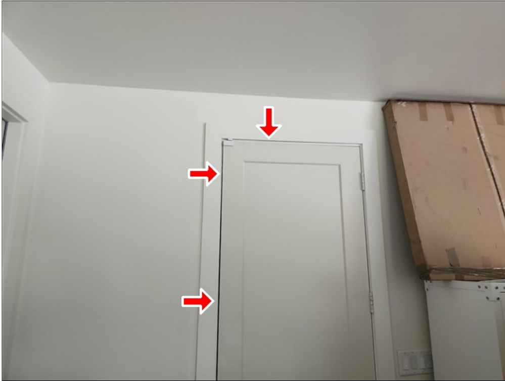
G. Excessive air gaps at exterior door in garage
