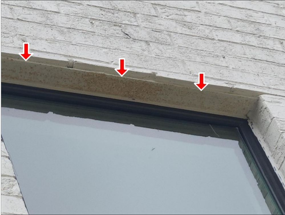
E. Photos showing steel lintels above windows rusting
