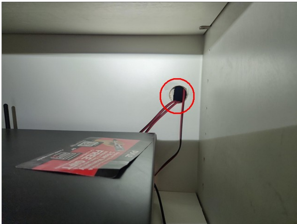
E. Second level game room closet has large hole in wall that should be sealed
