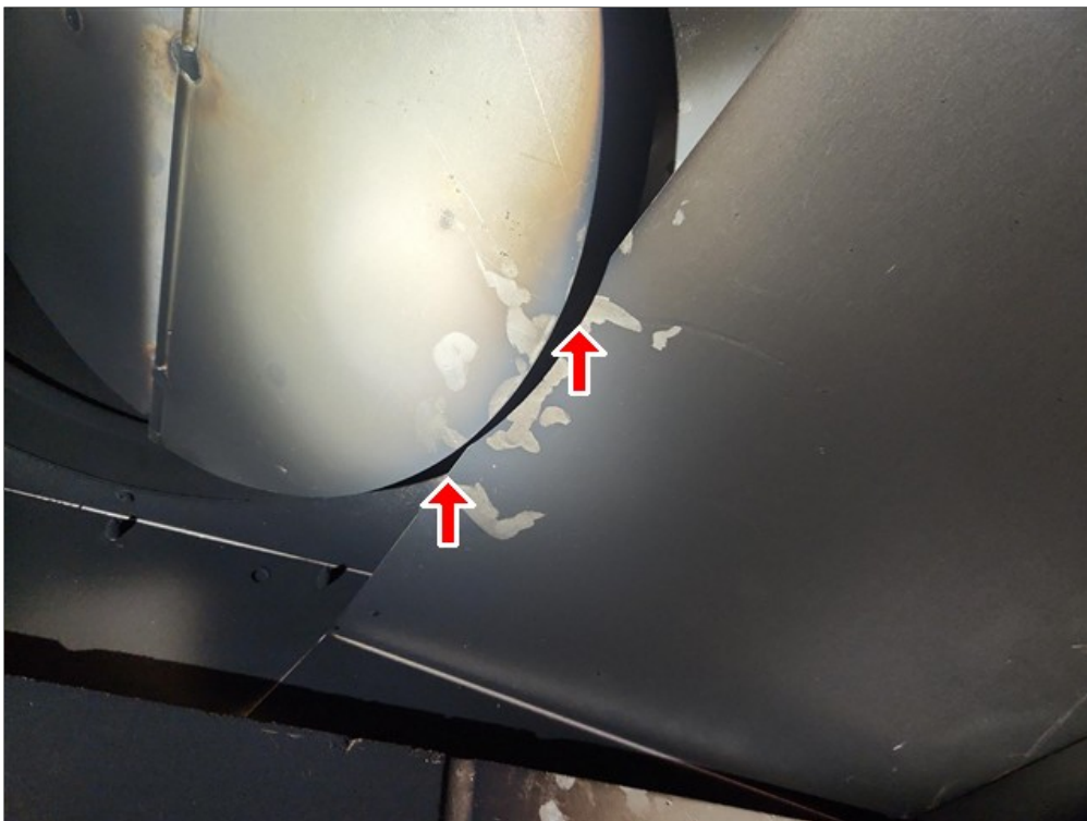
J. Damper being blocked by part of metal fireplace frame
