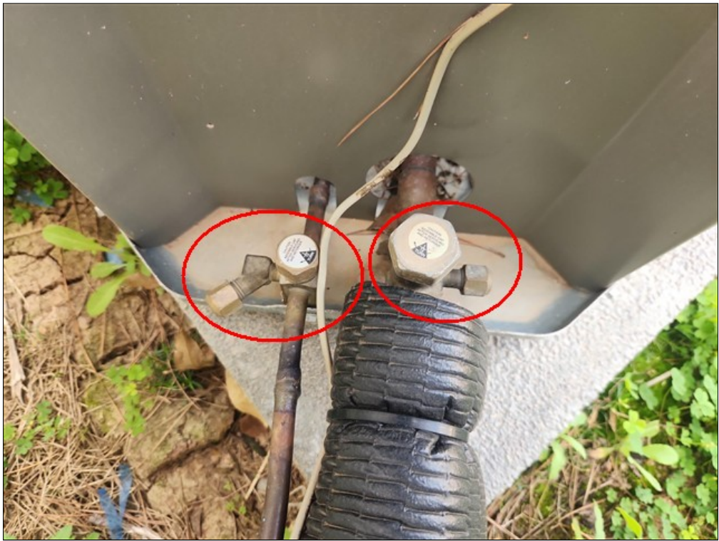
B. Missing locking caps at refrigerant ports
