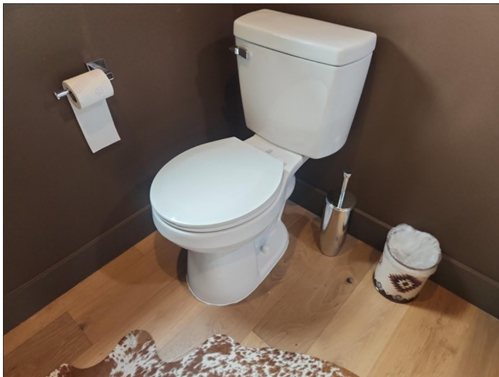
A. Toilet loose at floor
