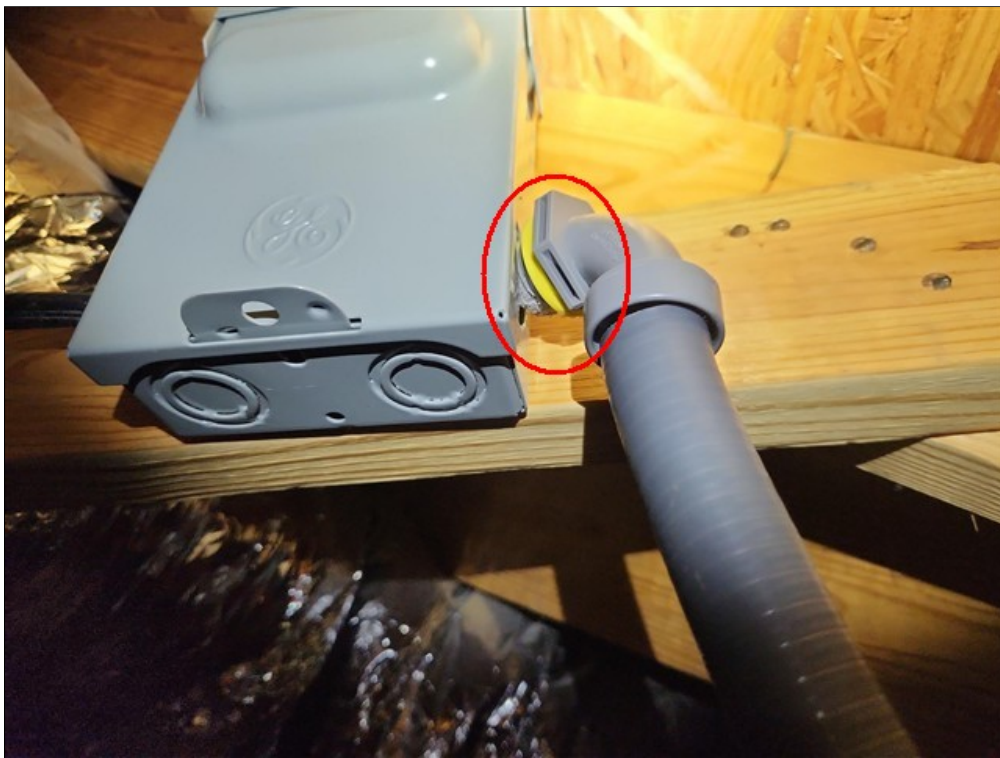
B. Conduit serving wiring to disconnect is detached from disconnect housing
