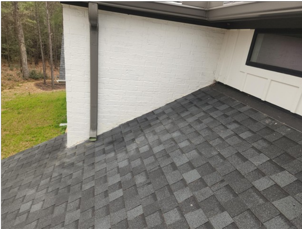
C. Photos of roof to brick wall transitions where flashing was not visible
