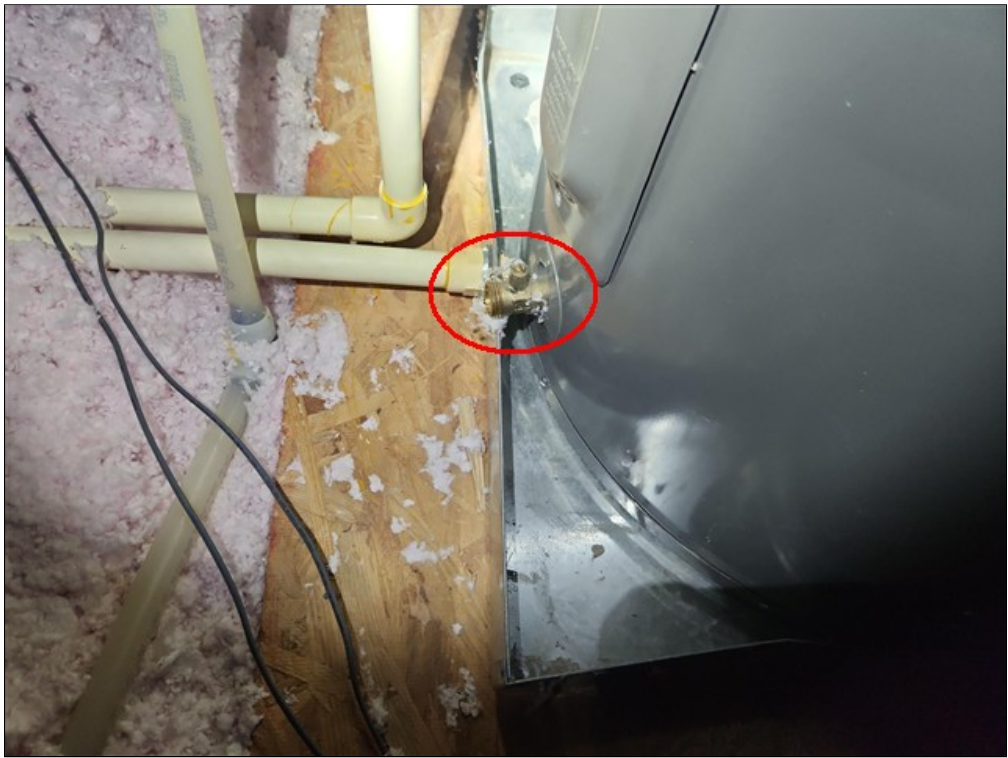
C. Drain valve extends over safety pan
