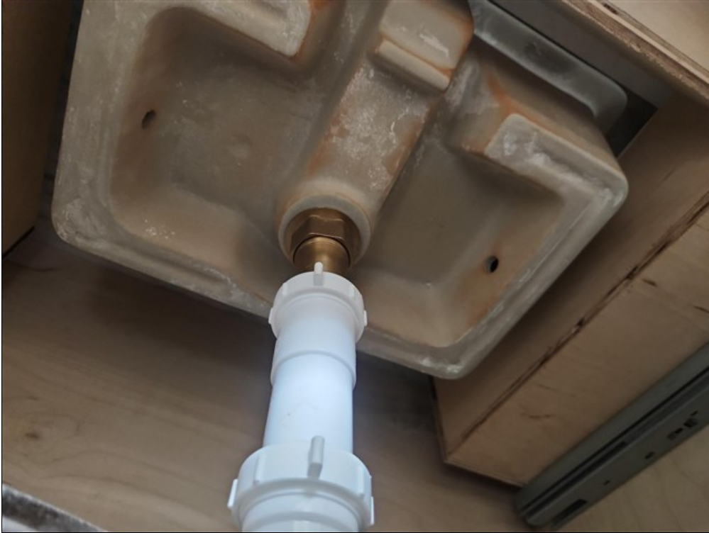
A. Undermount sink missing braces/clips
