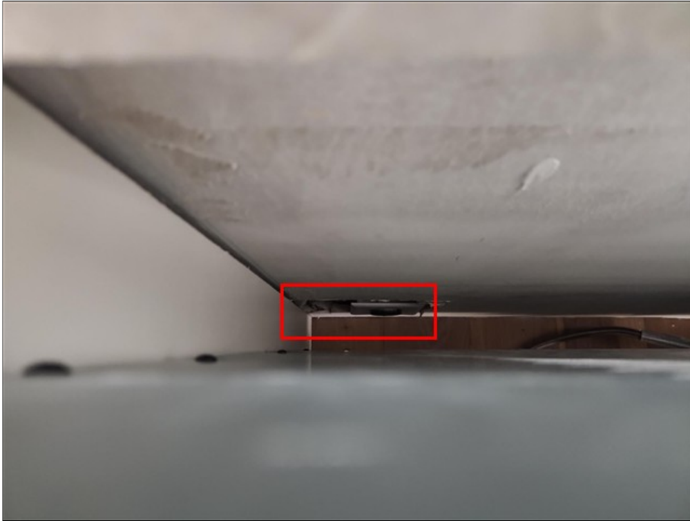
E. Excessively large hole in wall around receptacle behind range
