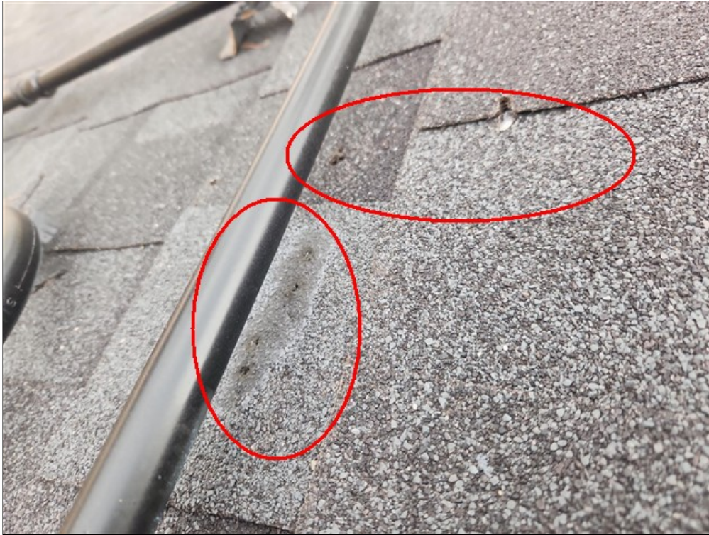
C. Photos of damaged shingles (holes in shingles)
