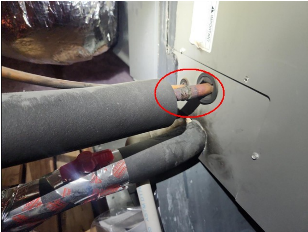
B. Mastic improvements needed where refrigerant line enters evaporator case
