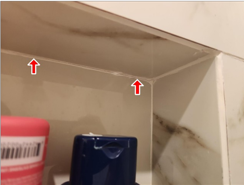
A. Caulking improvements needed at shower walls
