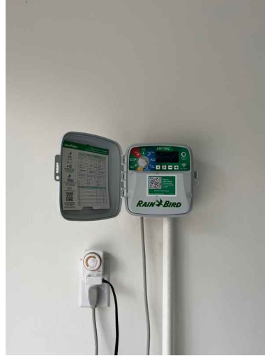
Sprinkler system control panel, located inside the garage
