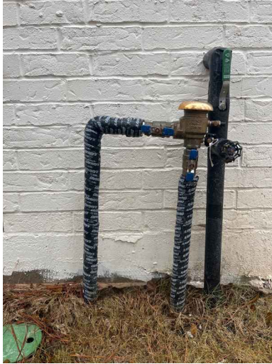
Sprinkler system backflow preventer, located left side of home
