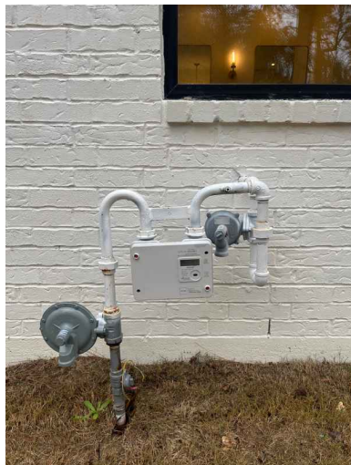
Natural gas meter, located left side of home
