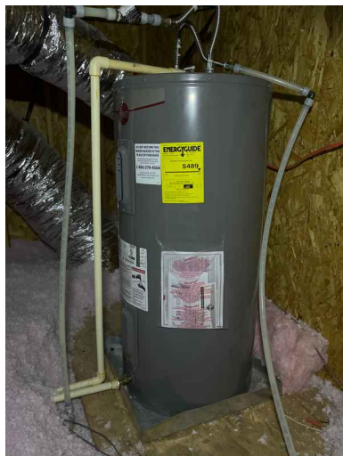
50 gallon electric water heater, located in the attic above master
