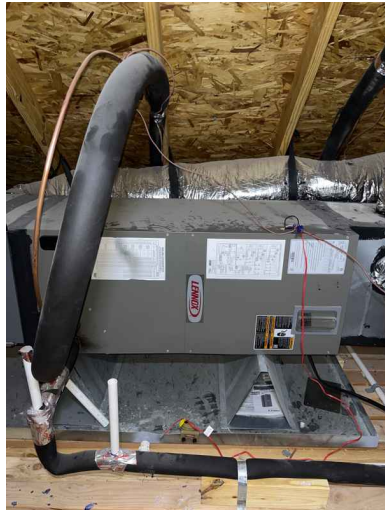
Electric furnace unit #1 (Left side of home)
