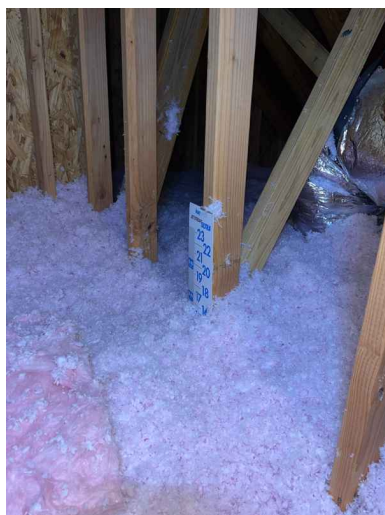
16 inches fiberglass insulation
