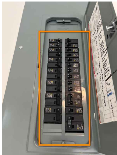
Main service panel
