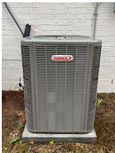
HVAC Condenser unit #1 (left side of home)
