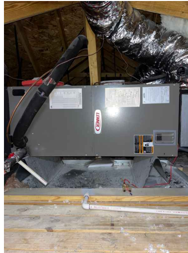
Electric furnace unit #2 (Right side of home)
