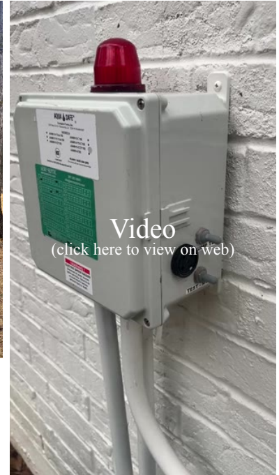
High water alarm functioning
