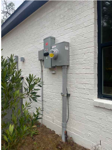
Below ground service and main service disconnect, located front left side of home
