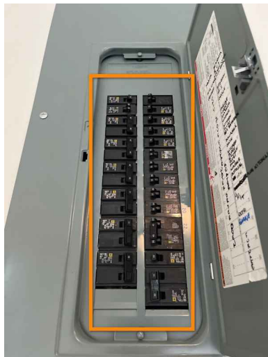
Main service panel
