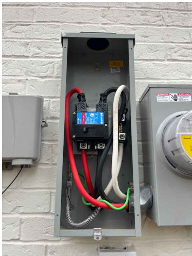
Main service disconnect, located outside, left side of home
