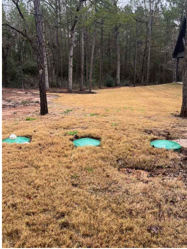
Septic system tanks, located rear of home
